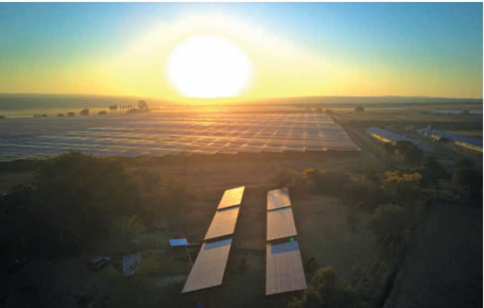
This solar plant, in the Brits area, is one of the first grid connected solutions which Eskom and NERSA approved.
